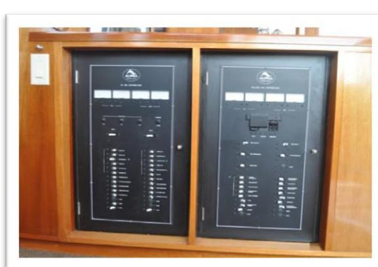
Main Electric Panels
